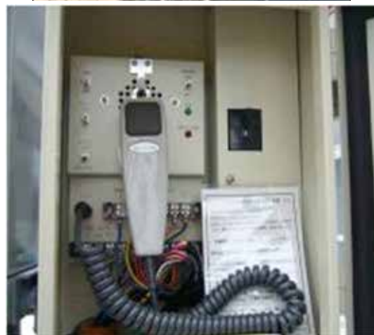
Photo 2.4.2 Information transmission Equipment for communication with local residents
